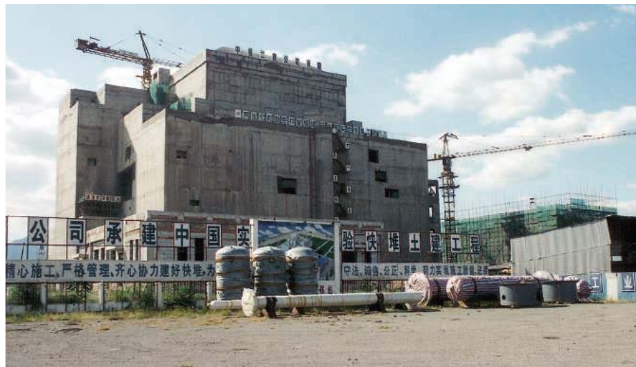
On the way. China has completed a building and workshop for its experimental fast reactor; the system is scheduled to be commissioned in 2008.
